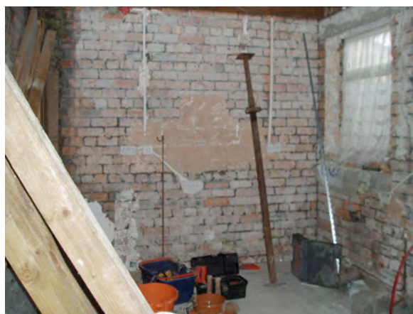
Example of damage caused by leaving a property empty
